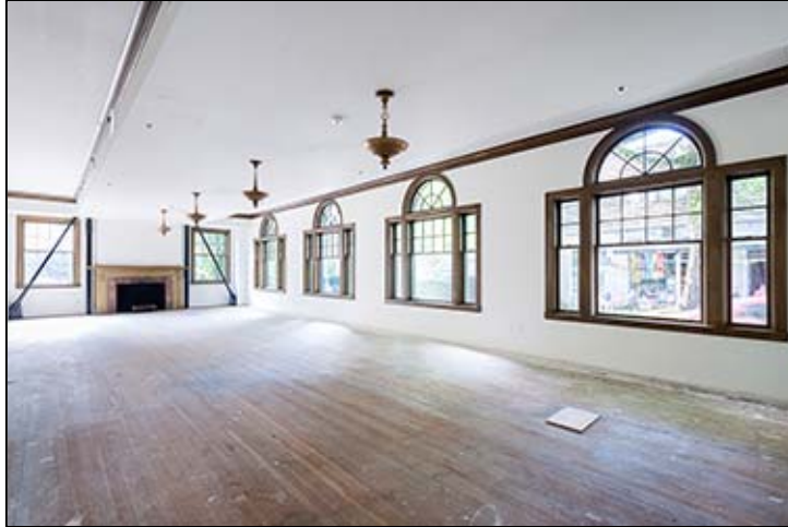
The lobby, “could be office space, could be a restaurant,” Shapiro says.
